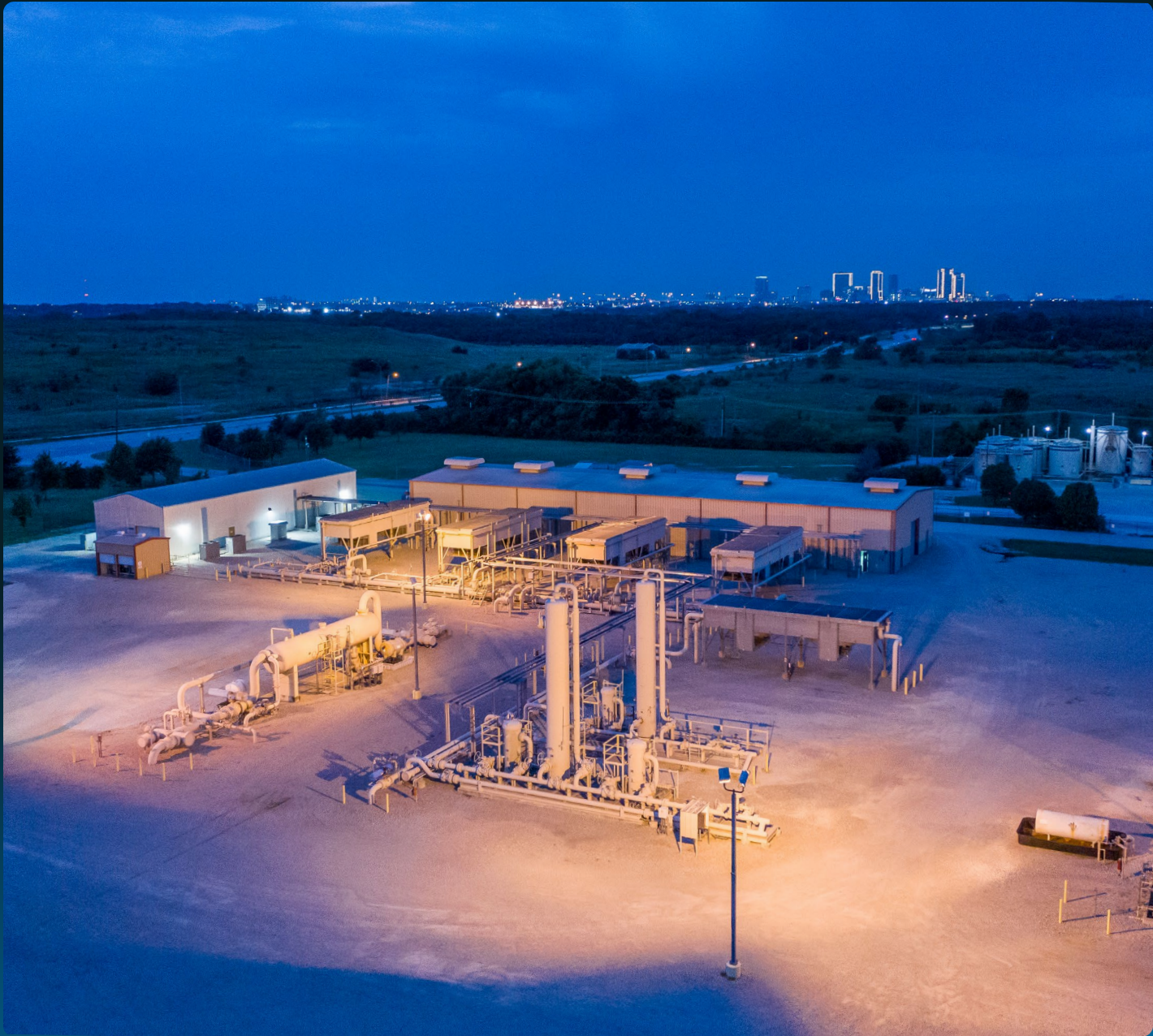
The Arc Park Compressor Station in Fort Worth, Texas.
